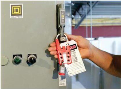
Group Isolation Device For Two Personnel Working on Pumps Each Authorized Personnel Working on Equipment Must Place Personal LOTO Lock
